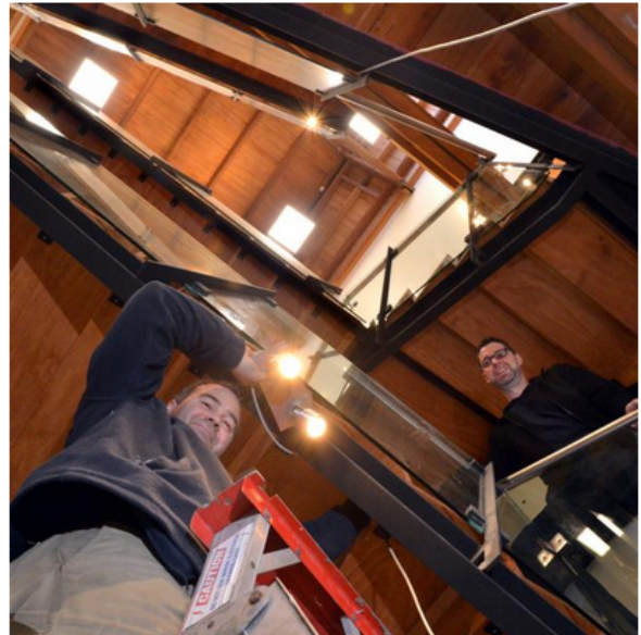
Winston Fenton (left) installs an LED light fitting in the Dunedin warehouse of ADInstruments owner Michael Macknight (right). Inset: The newly refurbished Donald Reid warehouse. Photo by Gerard O'Brien.
